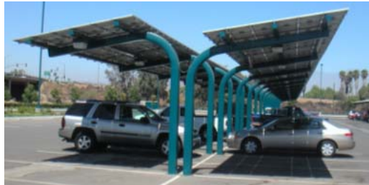
Photovoltaic Carport Structure at the La Sierra Metrolink.
